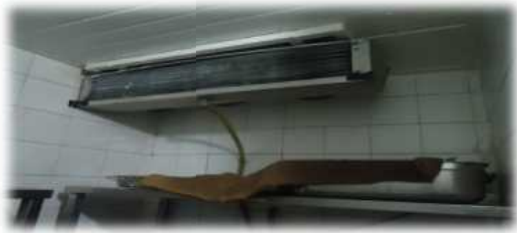
Fig 3. The air conditioning is old and maintenance-free.
