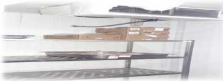
Fig. 4. The air conditioner be covered with ice because of extreme cooling.
