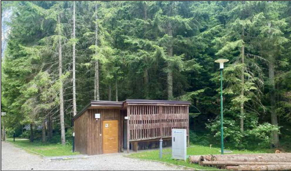
Figure 9: Wastewater treatment infrastructure in the Bijambare Protected Landscape. Biological treatment unit with a grease and oil separator located in the core tourist zone of the Bijambare Protected Landscape.
