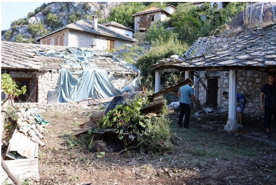
Fig. 5. The process of reconstruction and revitalization of the Madrasah in Počitelj Source: https://bljesak.info/magazin/religija/zapocao-proces-rekonstrukcije-i-revitalizacije-medrese-u-pocitelju/483851 (accessed: 4 December 2025)
